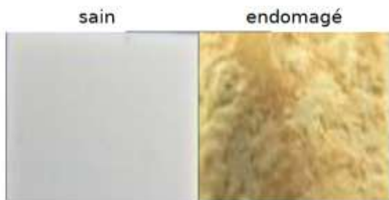
Figure 6. Photo de joint en silicone corrodé [12]
